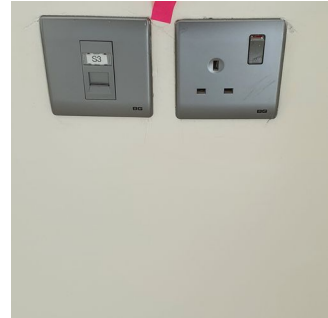
4. Electrical Switches and Sockets
