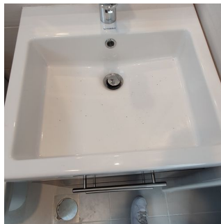
2. Wash Basin & Faucet
