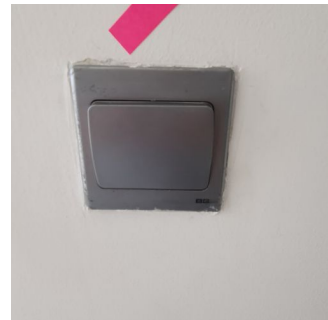
4. Electrical Switches and Sockets
