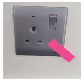
5. Electrical Switches & Sockets
