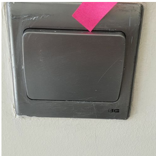
4. Electrical Switches and Sockets
