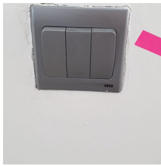
5. Electrical Switches & Sockets
