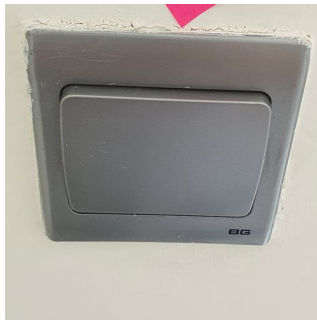
4. Electrical Switches and Sockets
