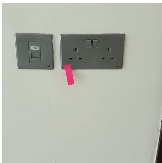
4. Electrical Switches and Sockets
