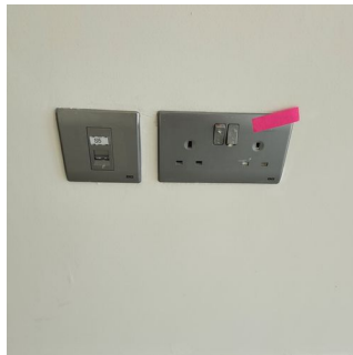
4. Electrical Switches and Sockets
