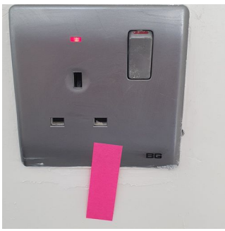
5. Electrical Switches & Sockets
