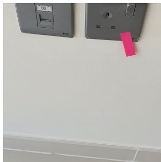
4. Electrical Switches and Sockets
