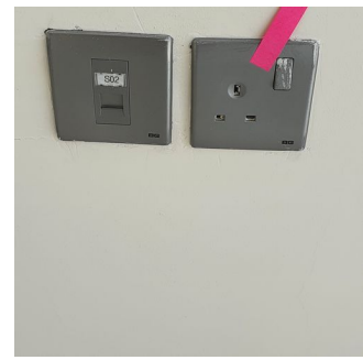
6. Electrical Switches & Sockets
