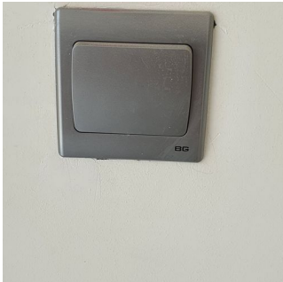
6. Electrical Switches & Sockets
