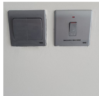
4. Electrical Switches and Sockets
